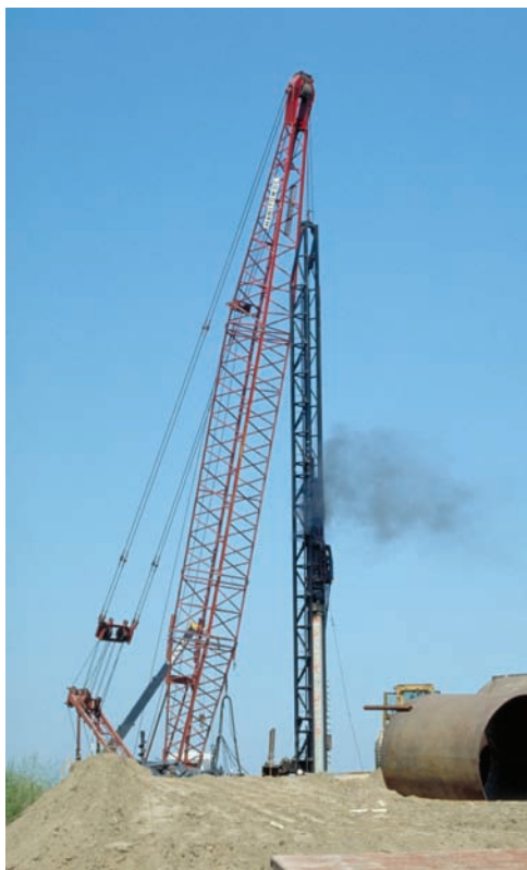
Photo 11.2 Steam alternately lifts a weight inside the pile driver and then propels it downward. This delivers a large impact load to the pile that is being driven into the ground.
