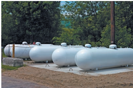
Photo 7.3 Cylindrical pressure vessels for liquid propane.
