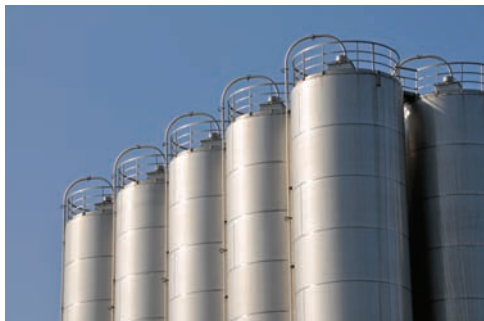
Photo 7.1 Cylindrical pressure vessels.
