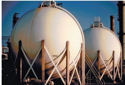
Photo 7.4 Spherical pressure vessels at a chemical plant.
