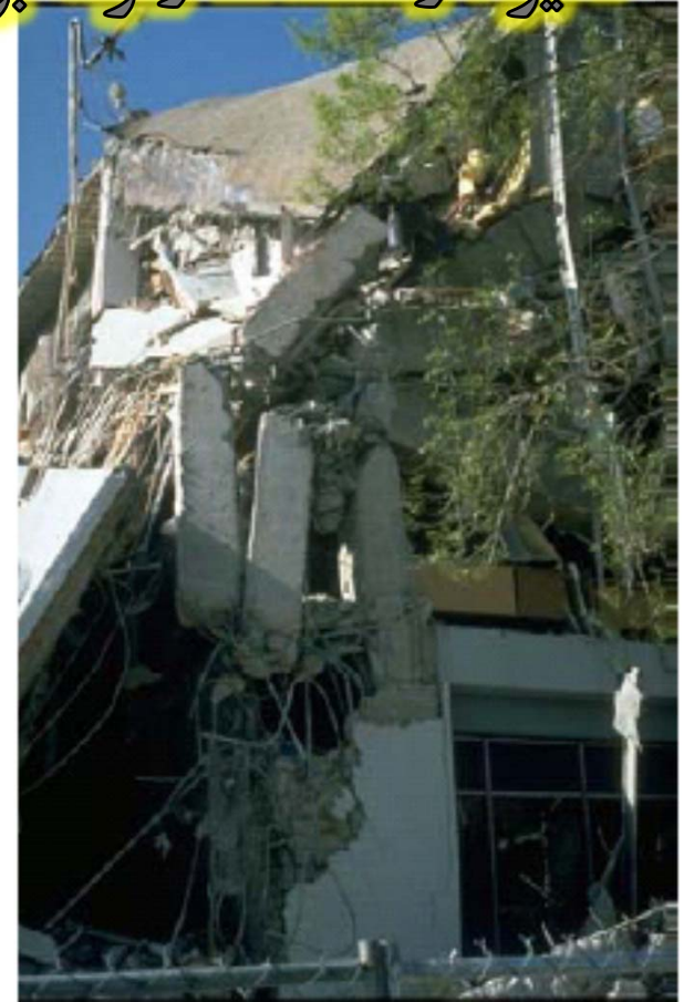
Figure 4 – Joint failures – Northridge earthquake
