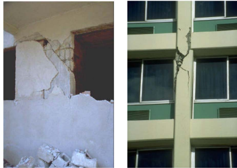
Figure 1 Column shear failures from (a) 1999 Kocaeli and (b) 1994 Northridge Earthquakes
