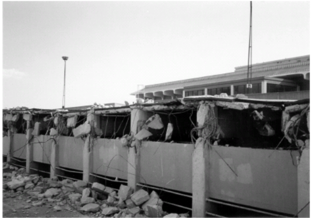
Figure 12-9. Collapse of concrete parking garage structure - October 17, 1989, Loma Prieta earthquake
