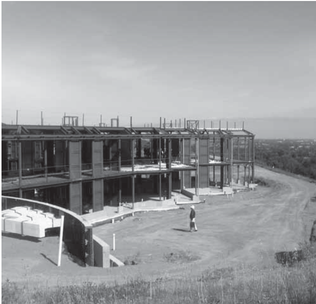
Fig. 1–26. Residential building with SPW in Los Altos, CA (courtesy of M. Eatherton, GFDS Engineers, San Francisco).
