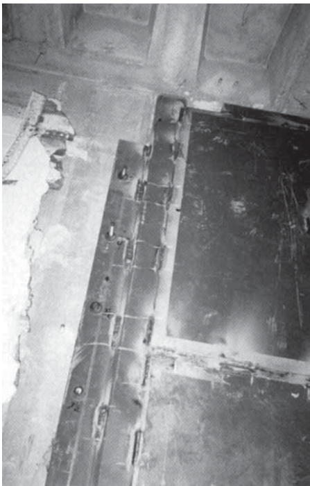
Fig. 1-18. New steel plate shear walls (courtesy of KPFF Consulting Engineers, Portland, OR).
