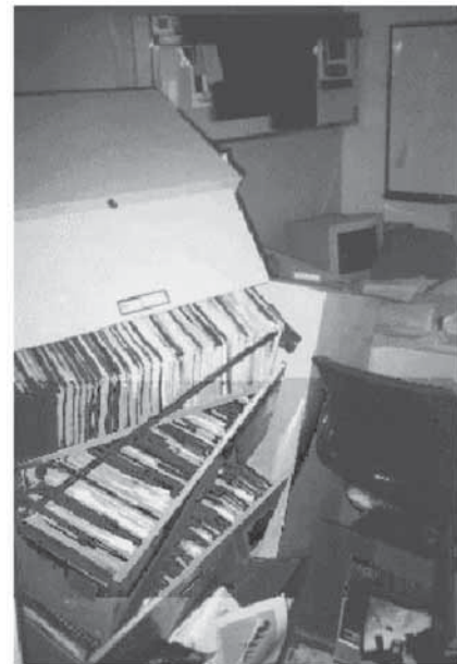
Fig. 1-15. Nonstructural damage in Olive View Hospital due to 1994 Northridge earthquake (Naeim and Lobo, 1997).
