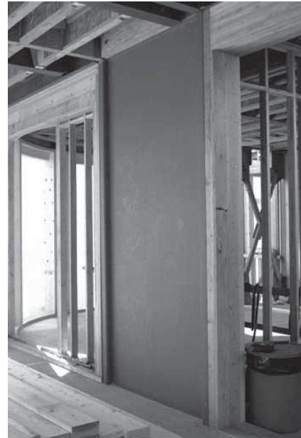
Fig. 1–27. SPW in four-story residence in San Francisco (courtesy of Jon Brody, Jon Brody Structural Engineers, San Francisco).
