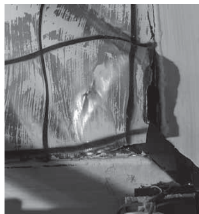
Fig. 2–16. Fracture of infill panel corner at 3.07 percent drift (Berman and Bruneau, 2003b).
