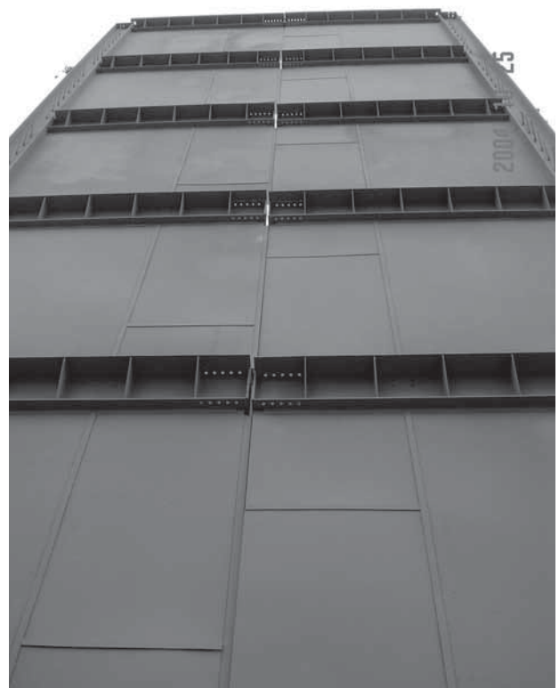
Fig. 1–32. Close-up view of wall at mid-span splice location, ING building (courtesy of Louis Crepeau and Jean-Benoit Ducharme, Groupe Teknika, Montreal, Canada).
