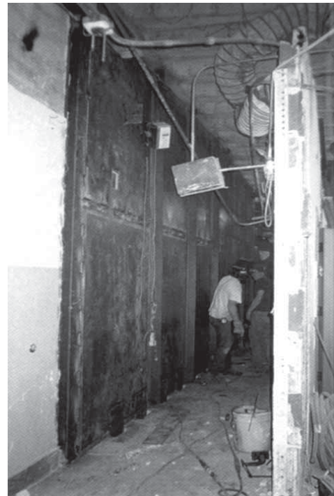
Fig. 1-17. Installation of new steel plate shear walls (courtesy of KPFF Consulting Engineers, Portland, OR).
