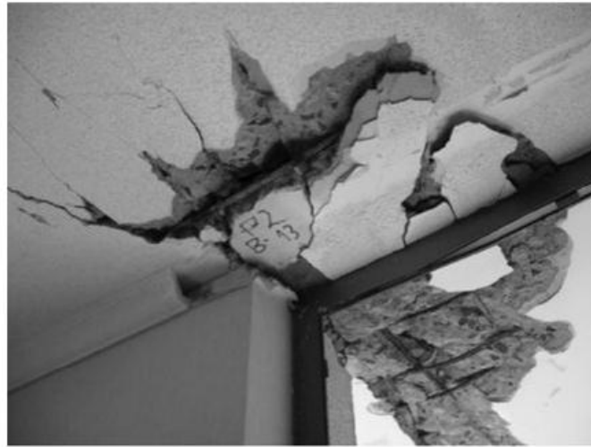
FIGURE 14.5 Punching shear failure of a slab acting as a coupling element between two structural walls, 2010 Chile earthquake. View upward toward ceiling showing wall boundary and damaged slab.
