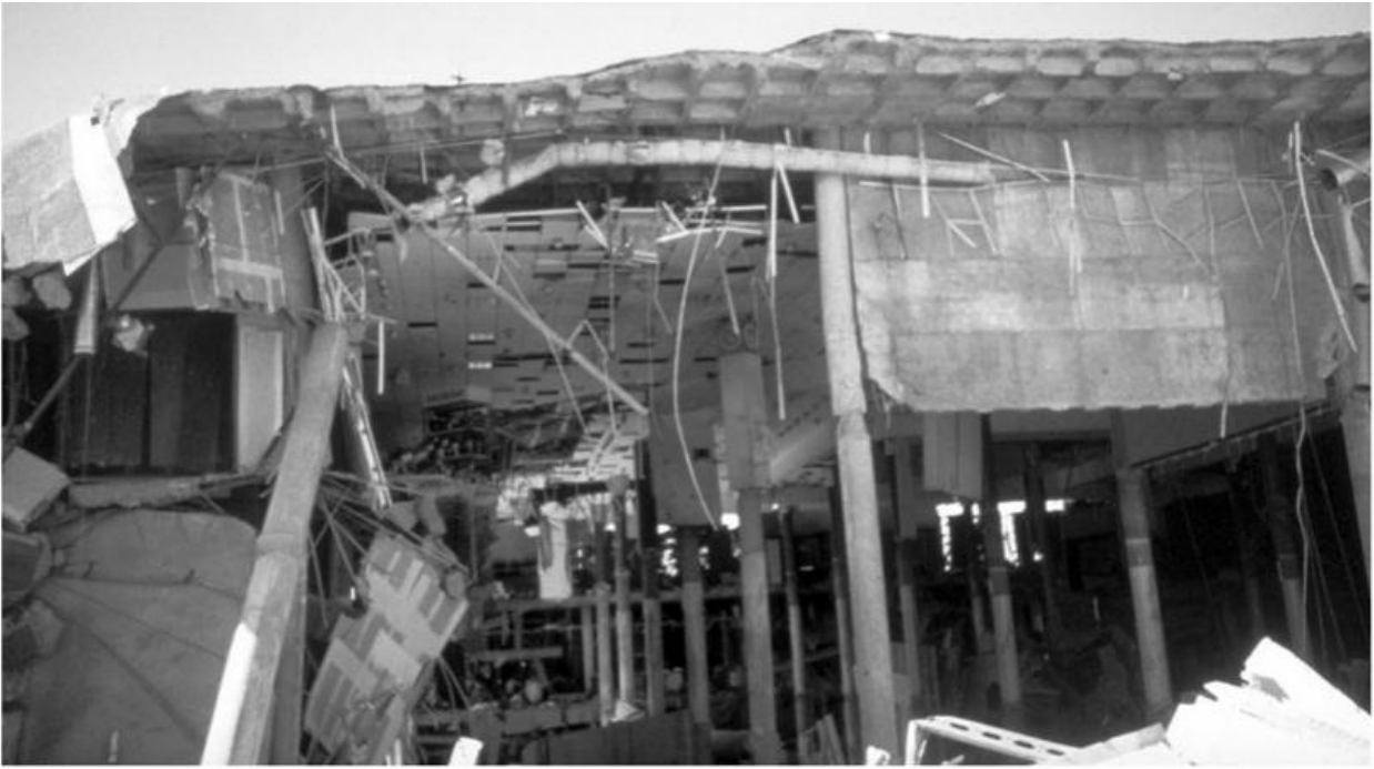
FIGURE 14.3 Damage and partial collapse of Bullock's department store in 1994 Northridge earthquake. (Used with permission from the National Information Service for Earthquake Engineering, University of California, Berkeley.)
