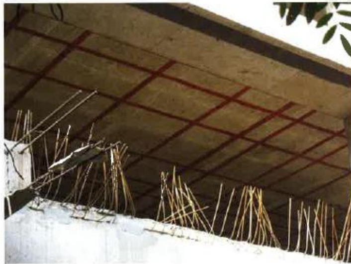
FIGURE 2.5.3A-2 Soffit of Slab is Painted to Show the Location of Tendons (Mumbai; P206b)
