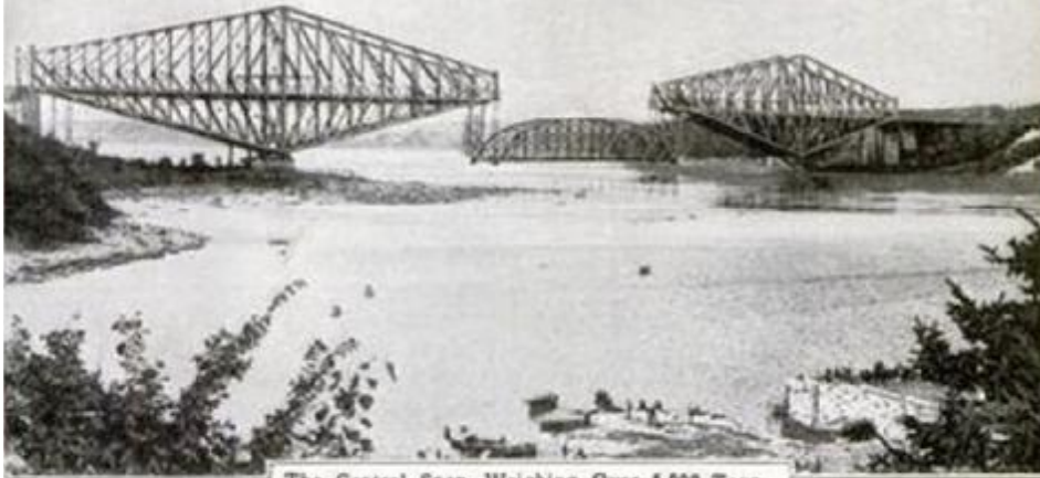
The Central Span, Weighing Over 5,000 Tons, being Raised by Practically the Same Method as was Employed Last Year, with Certain Added Precautions
