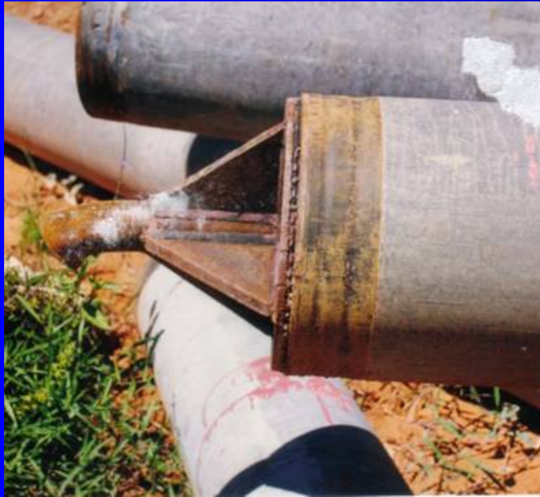
Defective pile shoe
