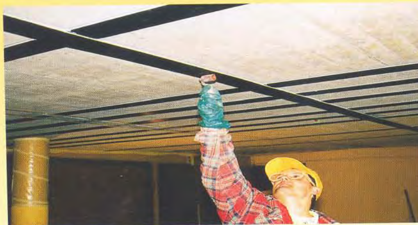
Strengthening of the reinforced concrete slab with the Sika® CarboDur® Plate System.
